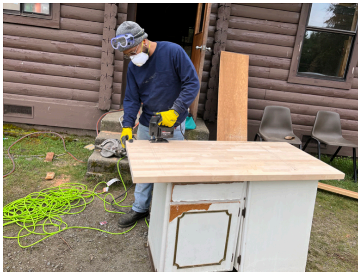
[Image description: A queer Black tradesperson wearing protective gear, sanding a kitchen table for a newly renovated cabin.]
